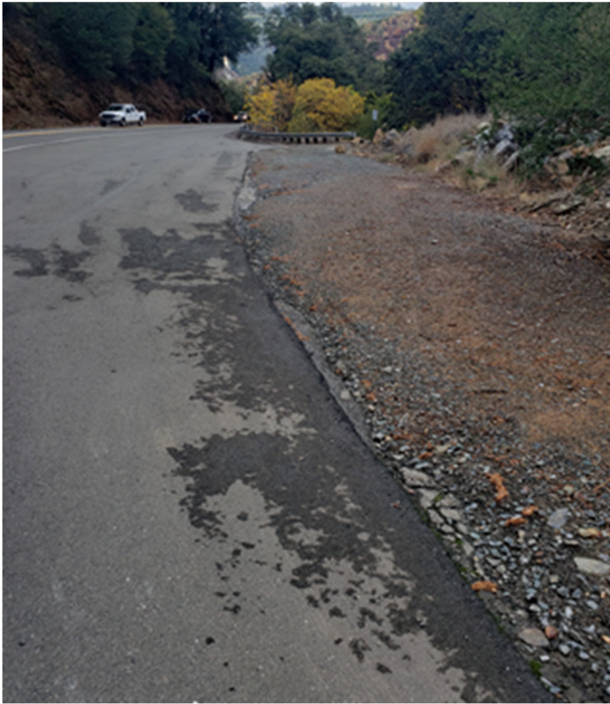
FIGURE 52: PHOTO OF SR 49 PARKING NEAR PM 35.5 EASTBOUND
